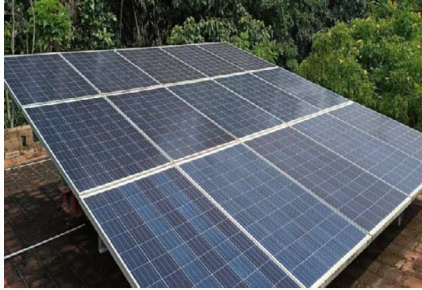
35 KW Solar Panel
